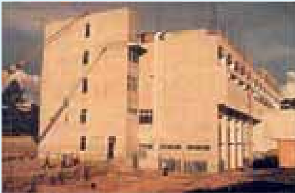
The construction of the first private hospital in Johor, KPJ Johor Specialist Hospital.
